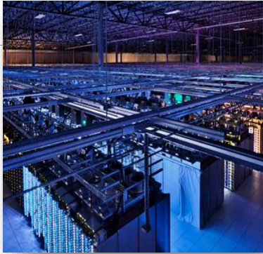
Cloud data center
